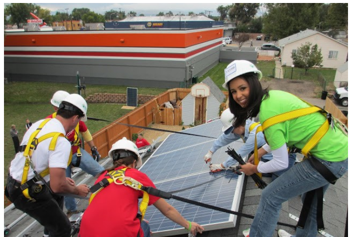
Fatima helps Wells Fargo volunteers and job training students install solar panels on her parents' home.
